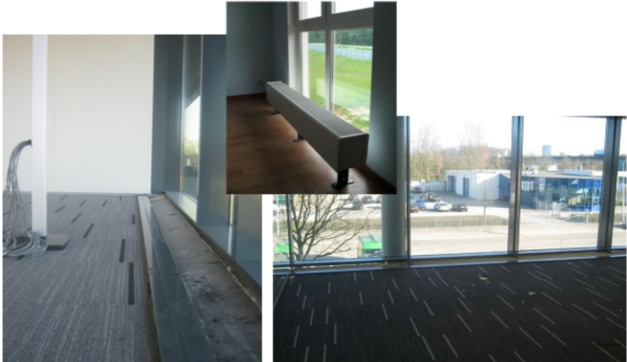
Designer radiators (inset) would have spoiled the look inside & out. ThermaSkirt saved the view and reduced costs.
