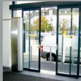
Installations for automatic sliding doors.
