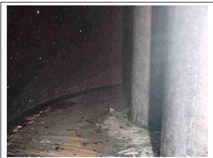
Same boiler looking to side, showing outer wall, heat exchanger floor and only a trace of accumulated scale.
