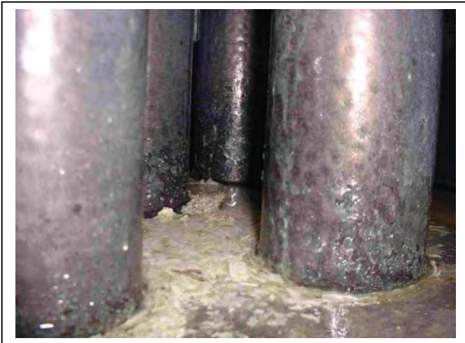
A closer view of limited 'flaky' scale in base of 60°C boiler unit.
