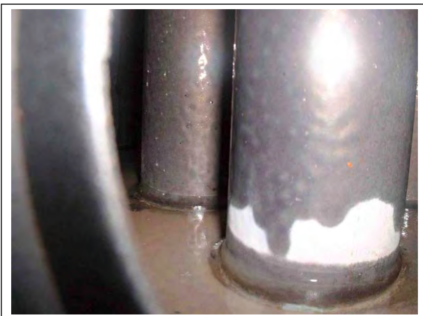
A view to one side shows even less effect on the rear flue and again no debris on the floor of the heat exchanger surface.
