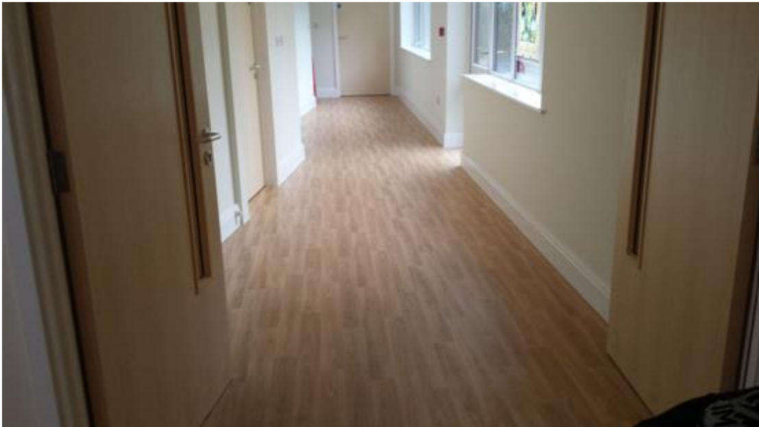
Corridors and gangways are kept clear of radiators by using ThermaSkirt throughout.
