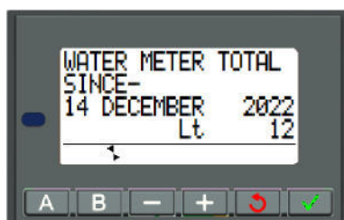
Water Consumption (since Installation)
