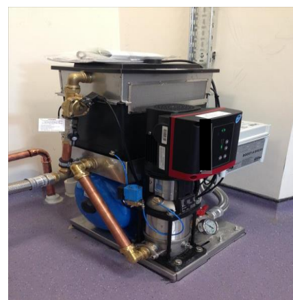
Fig 2: Storage cistern (break tank) supplying school laboratory
