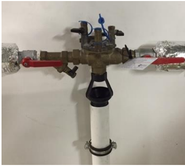
Fig 10: reduced pressure zone (RPZ) valve
