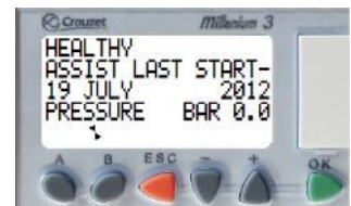
Date when the pump last started
